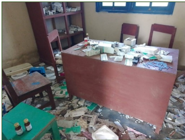
Fig. 5: Health Centre in the Suru-Suru District, Yahukimo Regency. Photo taken in August 2023
